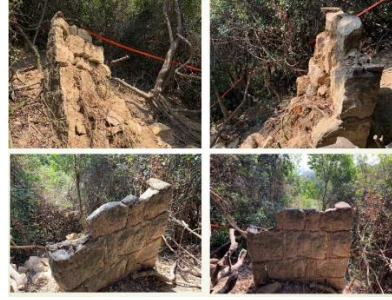
Figure 4b: The partially collapsed New North Mark in December 2019, revealing the rubble fill inside the cemented granite blocks. (Source: Daniel WONG)
